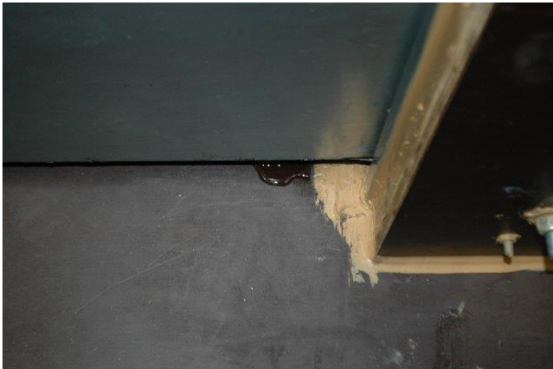
Photo C.3 Leakage under the test specimen 300 mm, water at the outside
