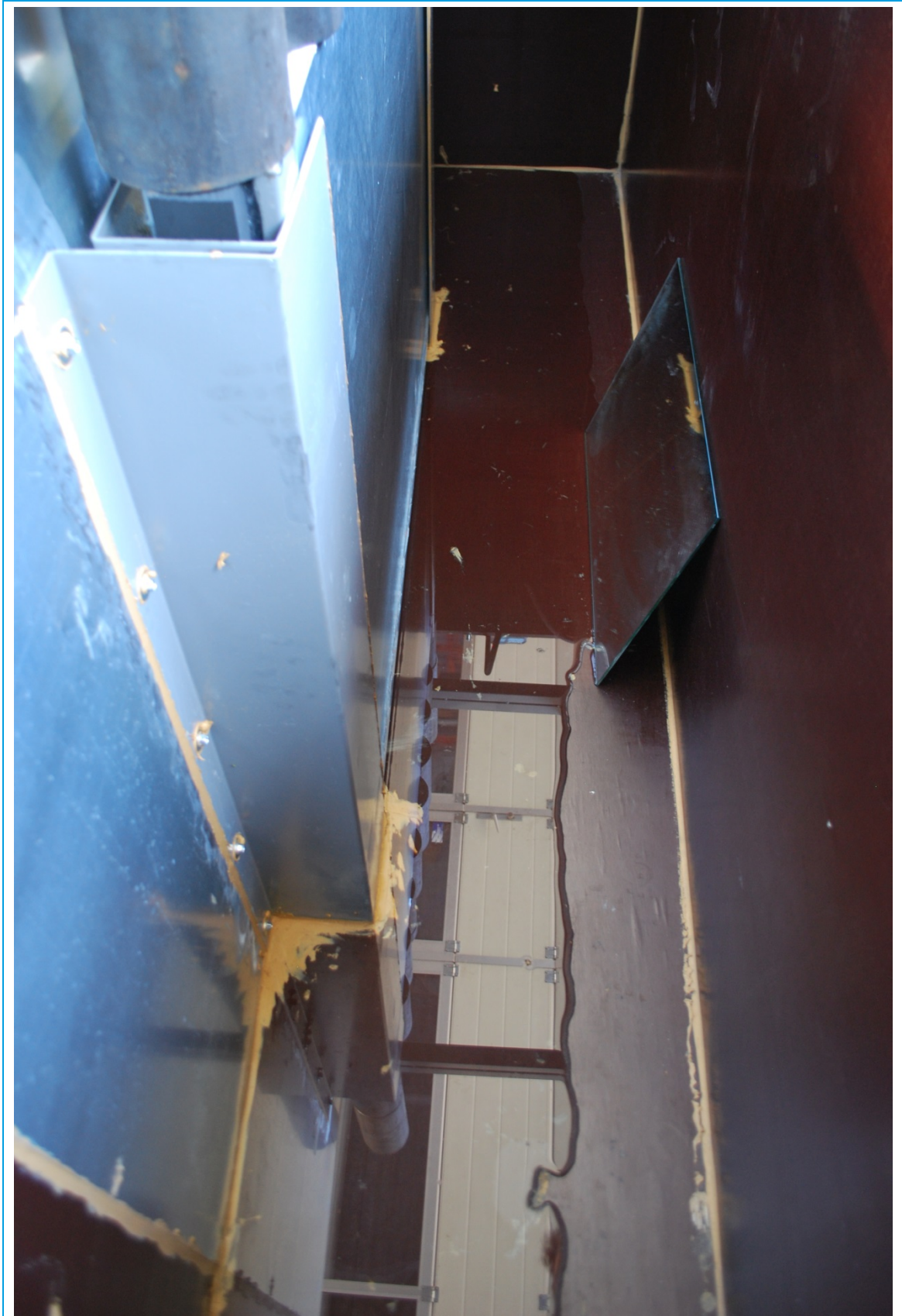
Photo C.9 Leakage under the specimen 1000 mm, water at inside
